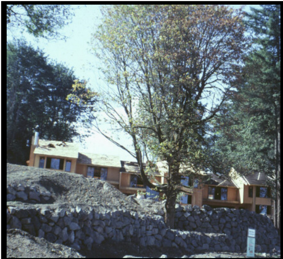
~ Caption: Root damage and dieback resulting from construction ~ Photo by: R.S. Byther
