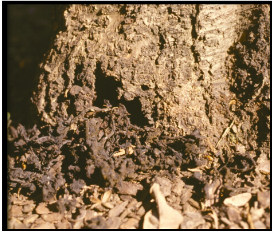
~ Caption: Peachtree borer damage at base of tree ~ Photo by: R. Van Denburgh
